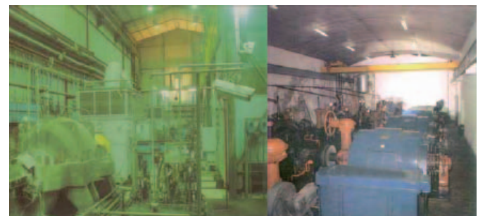
Fig. 6: On the right, the area of the -100 plant pumping station; on the left, the -200 plant pumping station.
